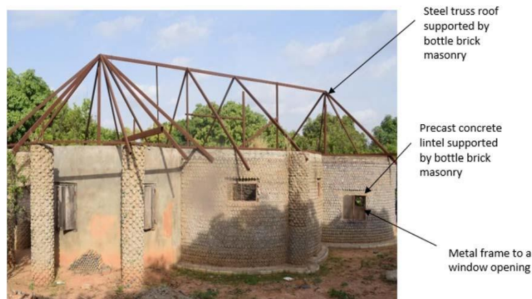
Figure 3. Plastic bottle bricks wall with steel truss roof and metal window frame (Edike et al., 2022)
