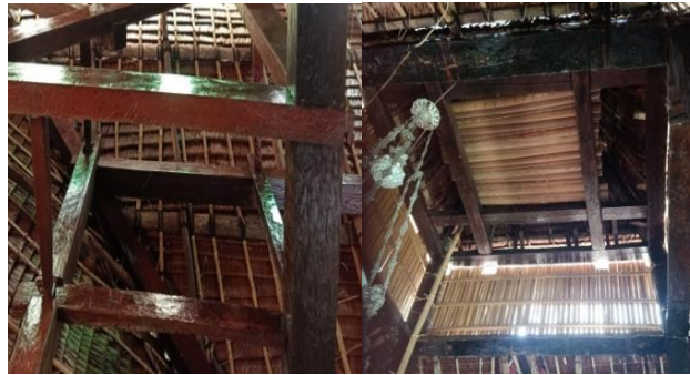
Figure 9. Cube shapes on the inside of the top roof and the first 4 corners of the roof
