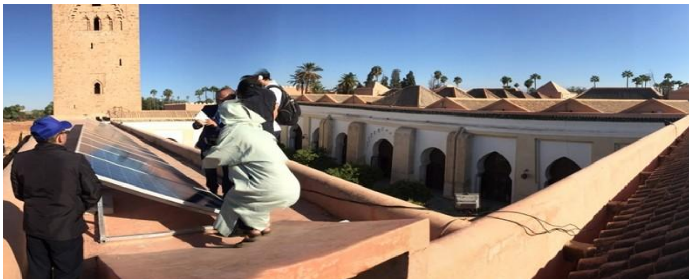
Figure 3. Solar Panel Installation on the Roof of Koutoubia Mosque, Morocco. (Source: Bentley/GroundTruth, 2017)
